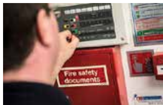
FIRE ALARM & FIRE FIGHTING MAINTENANCE
